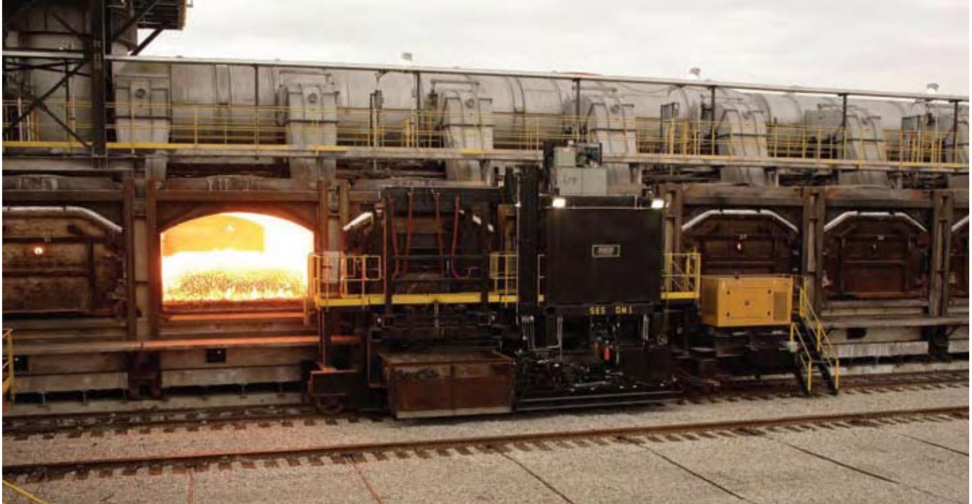
Fig. 20 Coke transfer car equipped with AP bearings
